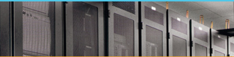
Integrated Racks And Cabinets
