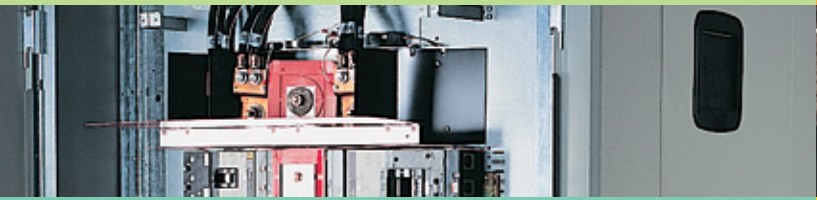
Power Conversion And Distribution
